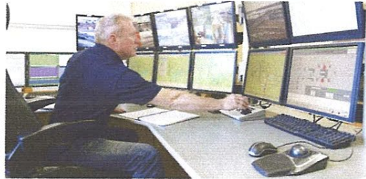
Figure 2.7: Fully equipped monitoring room for a CCTV system.
