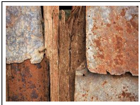
Figure I.6: La corrosion sous contrainte
