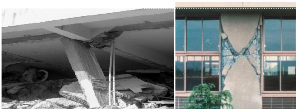
Figure I.16. Cisaillement des poteaux courts
