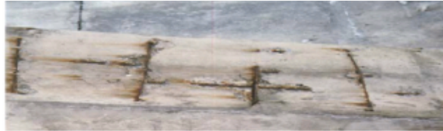
FigI.1: Corrosion des armatures
