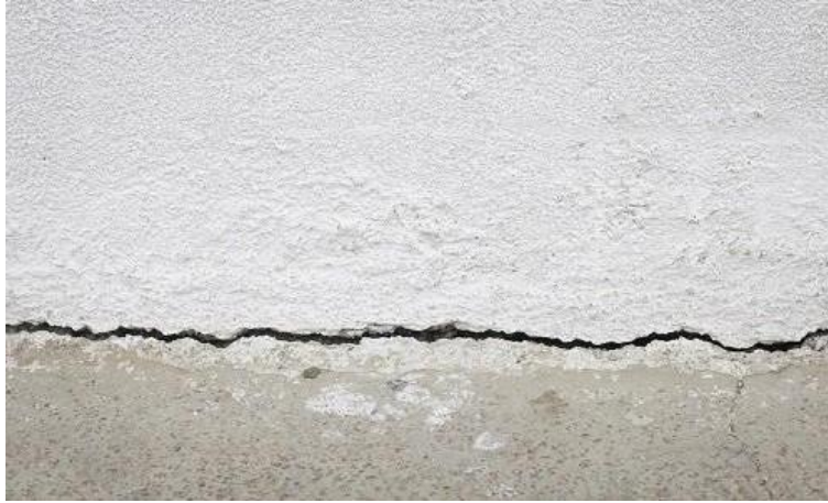
Figure II.19. Fissure horizontale de béton
