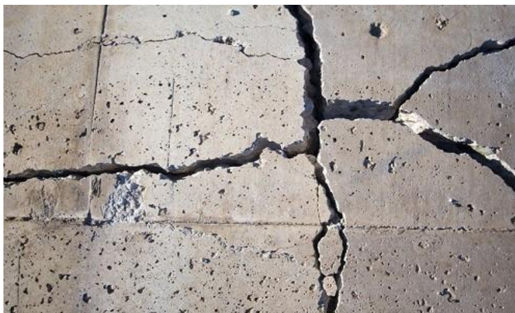
Figure II.22. Fissures de retrait-gonflement
