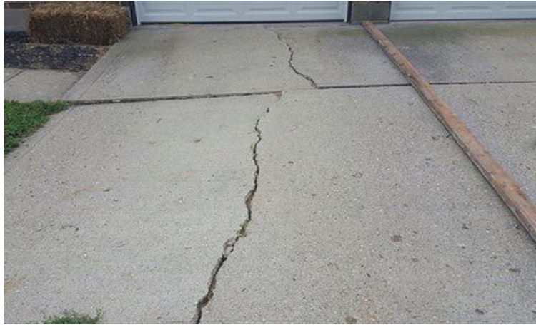
Figure II.21. Fissures de tassement
