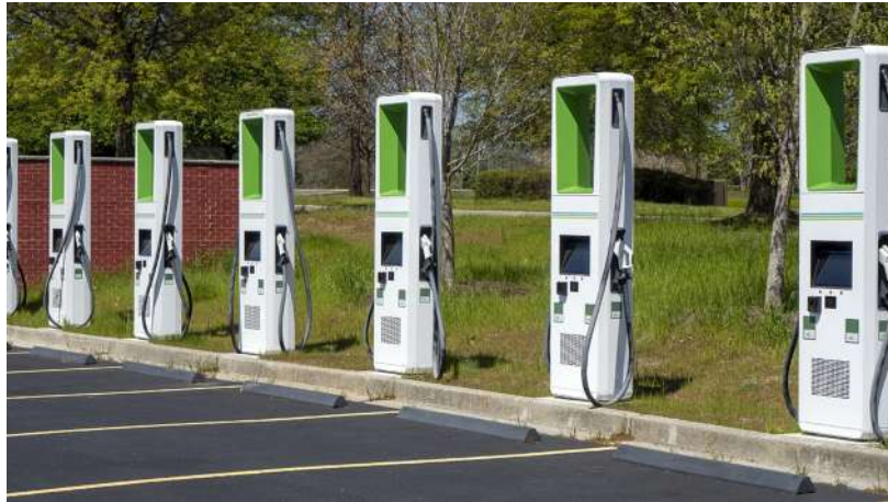
Figure 1.8. electric vehicle charging stations
