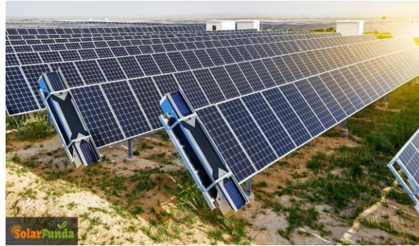
Figure I.16: solar panels Robotic cleaning.[20]
