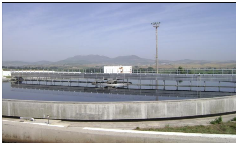
Figure 15. Bassin de clarification. (STEP Guelma, 2008).
