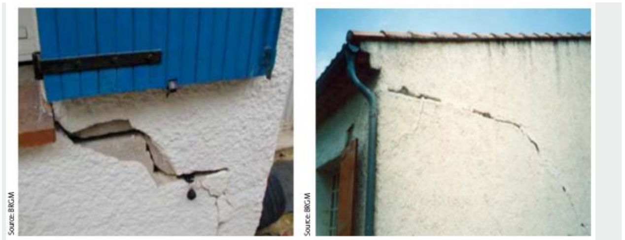
Figure I.12. Fissuration due au retrait-gonflement[39].
