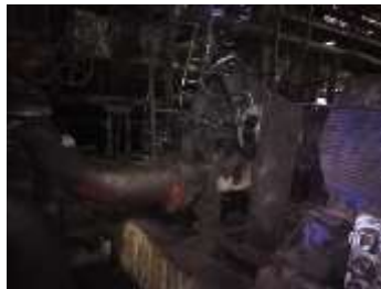
Figure.III.5 : La pompe G30
