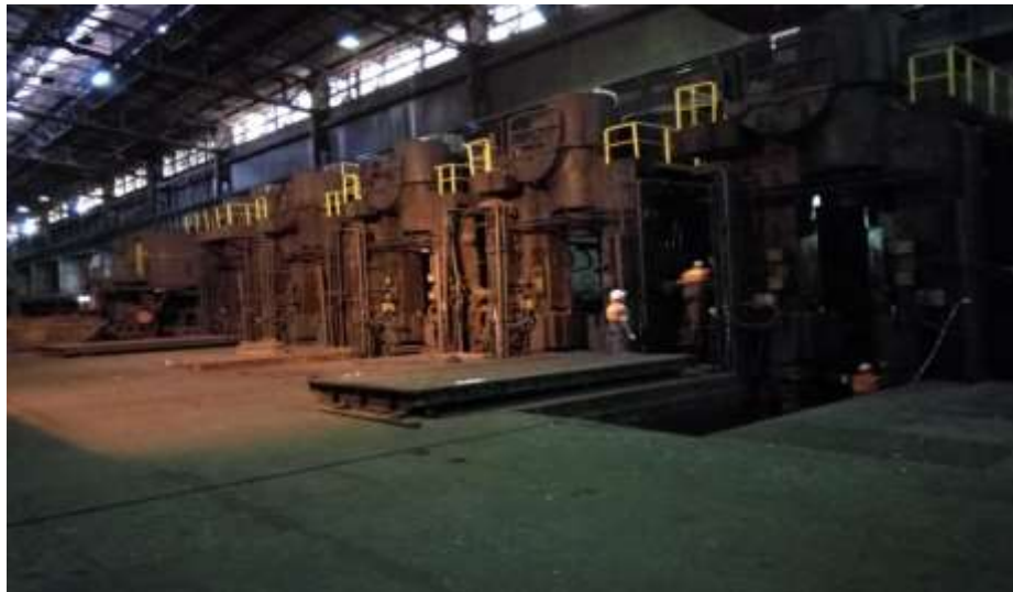
Figure.I.10: Train finisseuse (6 cages)
