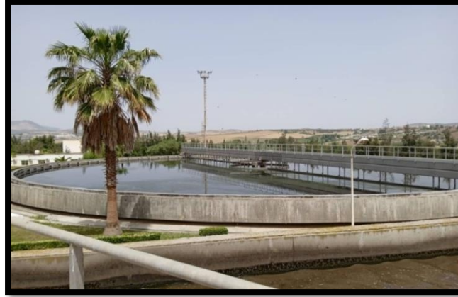
Figure II.7: Clarificateur (STEP Guelma 2022).
