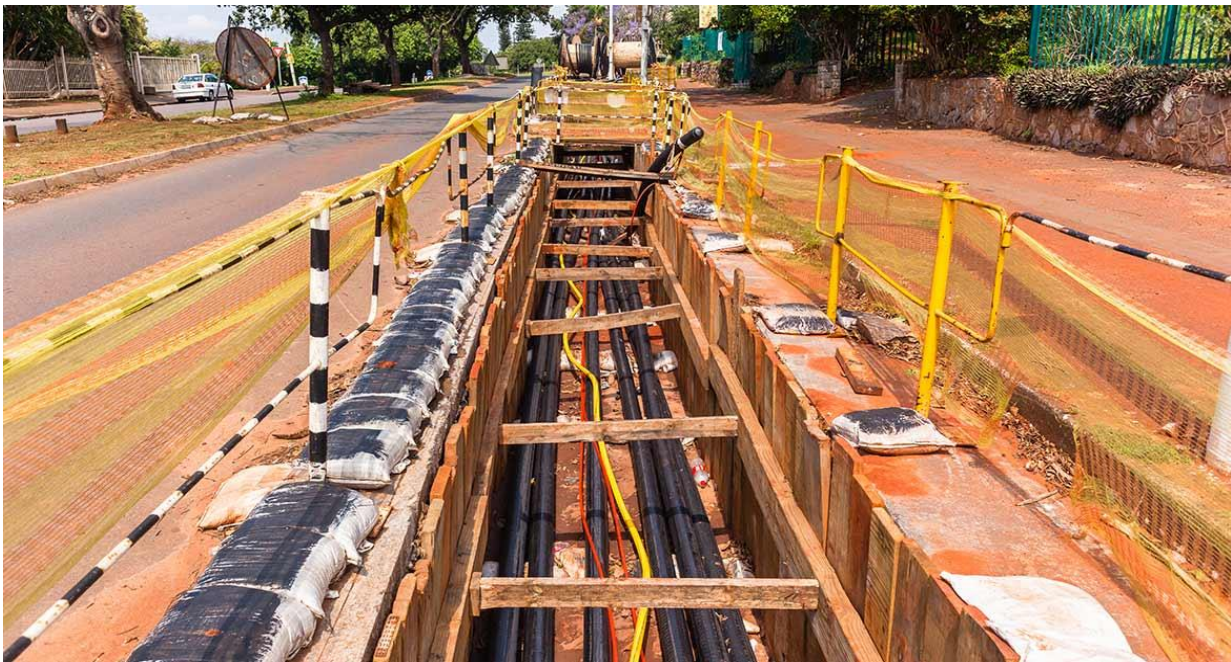
Figure I. 6: Câble HTA souterrain.
