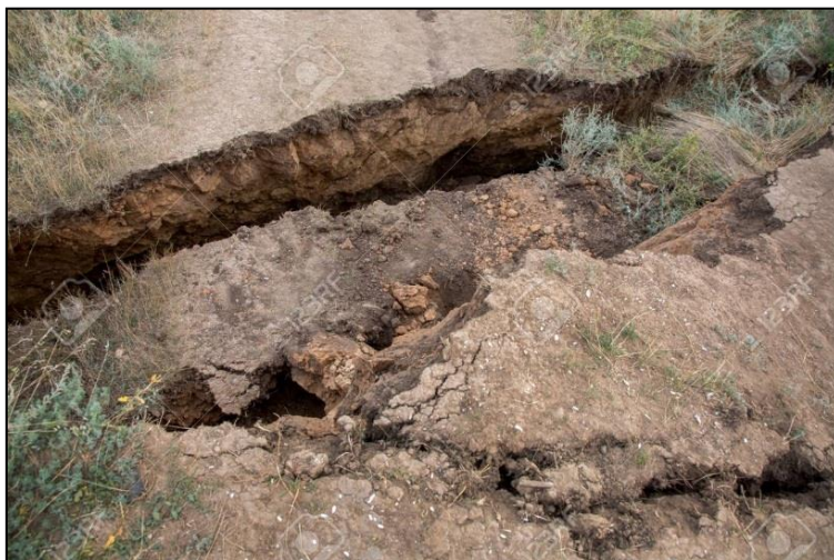
Figure 2.5 Fissure de tension
