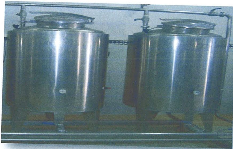
Figure III.4 : tanks de stockage
