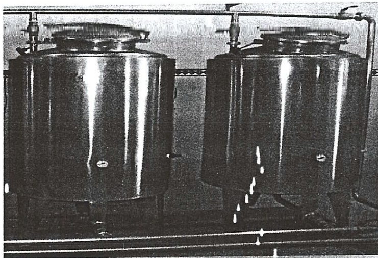
Figure 2.6 : tanks de stockage
