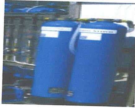
Figure 23: Photo d'une station duplex system A et system B.
