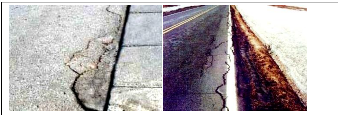
Fig.III.10: Fissures de rives
