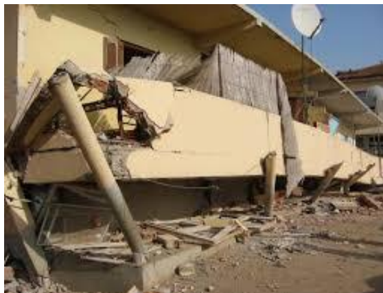
Fig 3.1. Collapse of Reinforced Concrete Structure in Boumerdes (2003) Earthquake Due to Weak Foundation Design.
