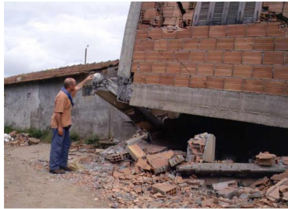
Fig 3.2. Column-Beam Failure Due to Insufficient Seismic Detailing in Zemmouri During the Boumerdes (2003) Earthquake [39].
