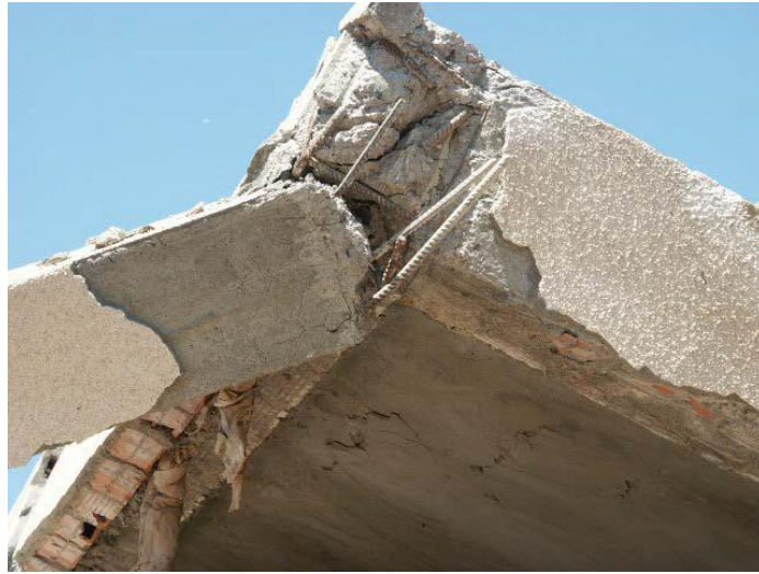
Fig 3.6. Shearing of Corner Column Due to Lack of Transverse Confinement and Poor Seismic Detailing: Example of Non-Compliance with Seismic Codes.
