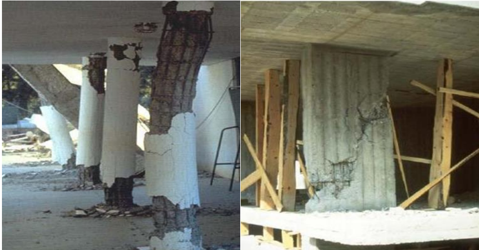
Fig 3.13. Failure of Vertical Load-Bearing Elements under Seismic Loading [43].
