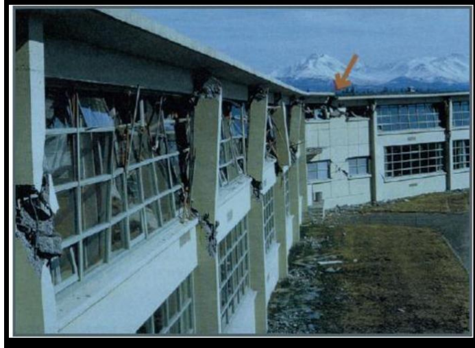
Fig 3.3. Damages to Roof Diaphragm at Re-Entrant Corner of West Anchorage High School During the 1964 Earthquake [40].
