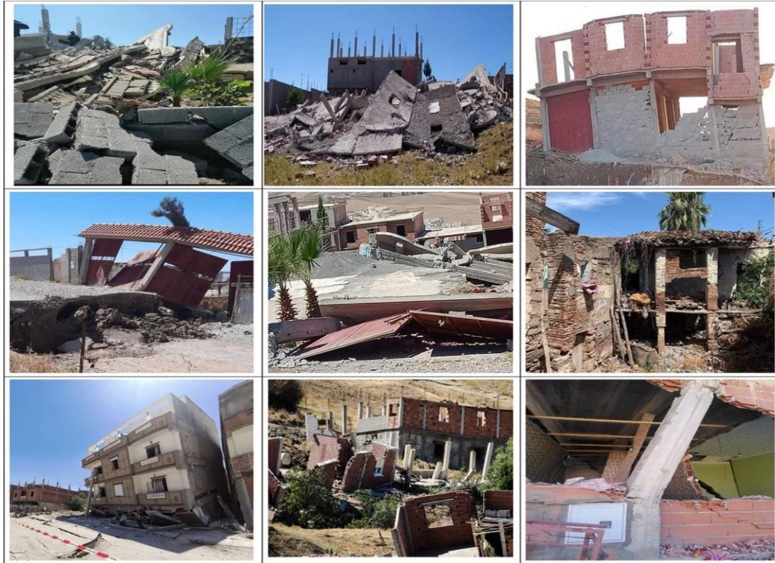
Fig 2.6. Structural damage due to liquefaction (Mila City, August 7, 2020).
