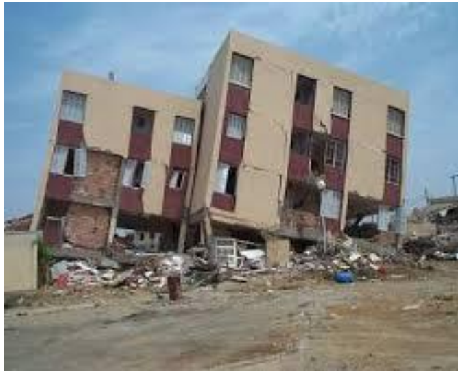
Fig 3.5. Foundation Failures and Structural Settlement in RC Buildings During the El Asnam (1980) Earthquake [15].
