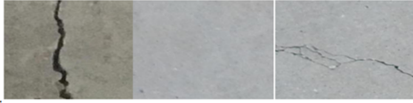
FIGURE 3.4: Some Pictures from dawgsurfacecrackssag Data [71, 72]
