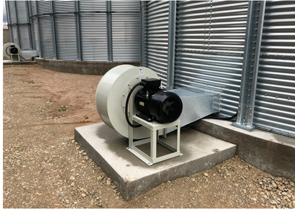
Figure 1.6: Modern Silo with Aeration Systems
