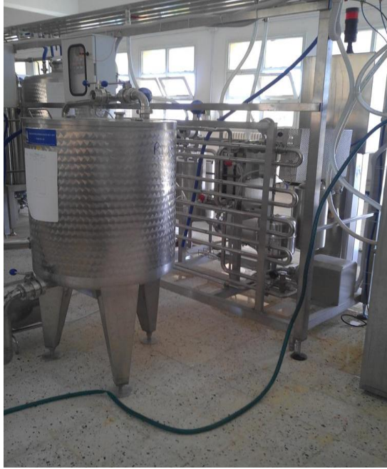
Photo 10. Tank de stockage
