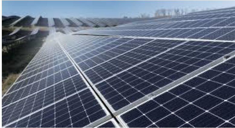
Figure II.5. Photovoltaic solar panels [44]
