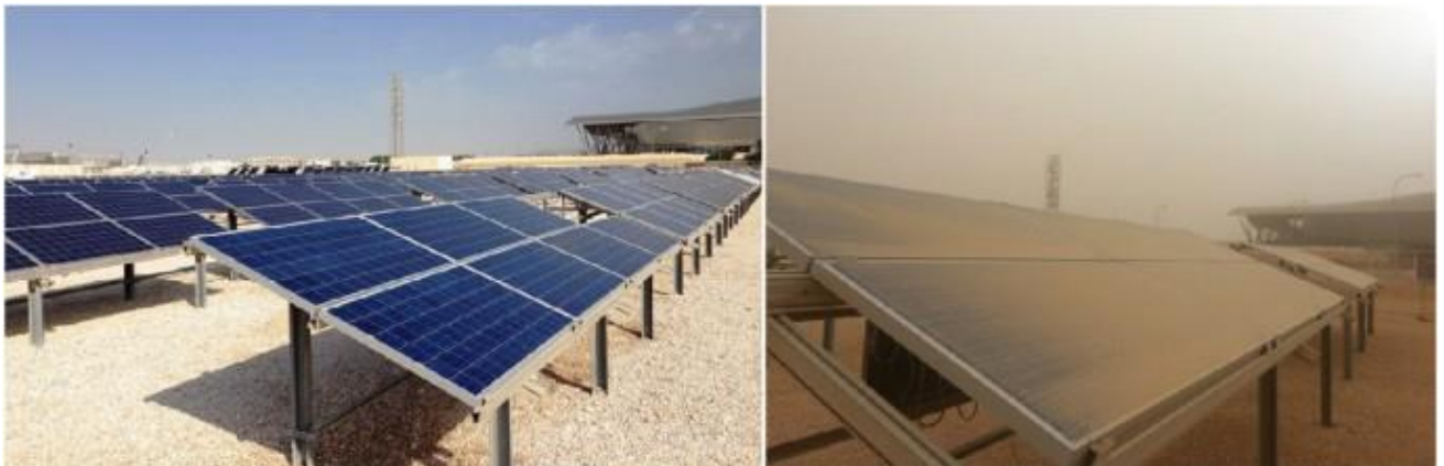
Figure II.8. Clean solar panels vs dirty solar panels [51]
