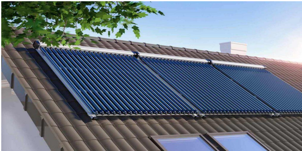
Figure II.3. Solar thermal panel [42]
