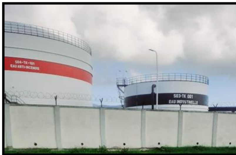
Figure II.2 : Stockage du Condensat
