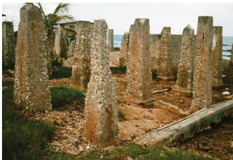
Figure I-7. Effect of sulfate-rich soil on concrete (concrete spalling) [16].
