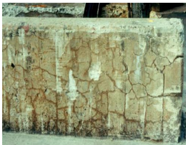
Figure I-5. Map cracking due to an alkali-silica reaction [14].
