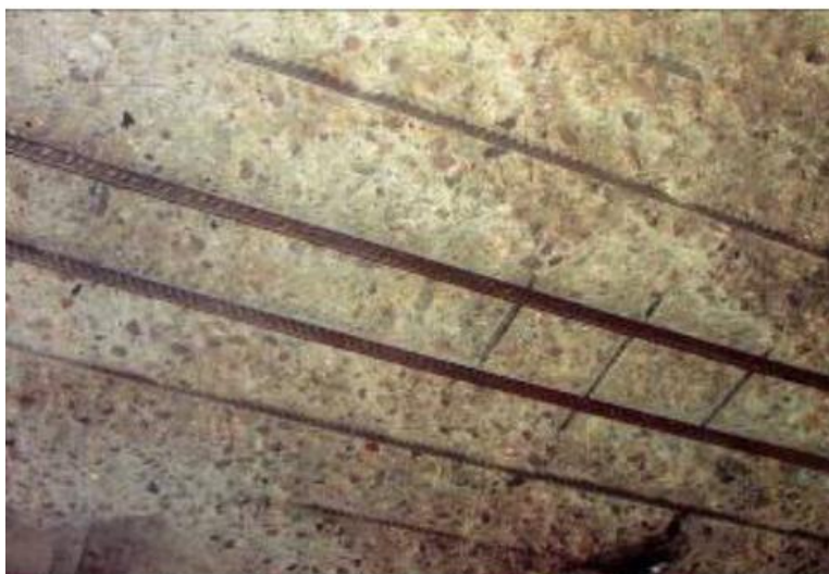
Figure I-4. Spalling in RC slab exposed to fire [13].
