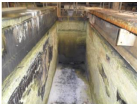
Figure I-6. tank damage containing hydrochloric acid [17].
