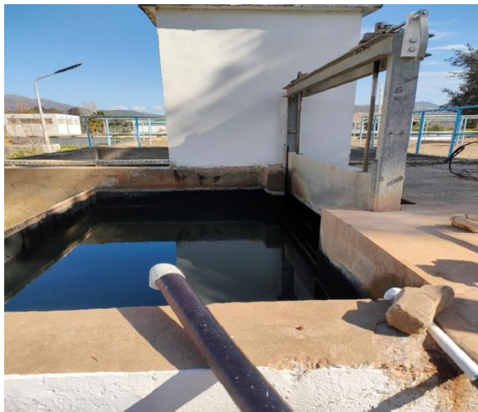
Figure III.1: Bassin de pré-chloration
