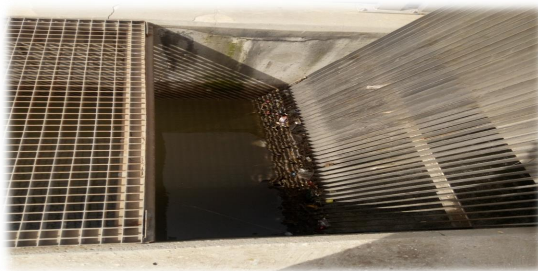
Figure. II.2.dégrillage (STEP Guelma 2021)
