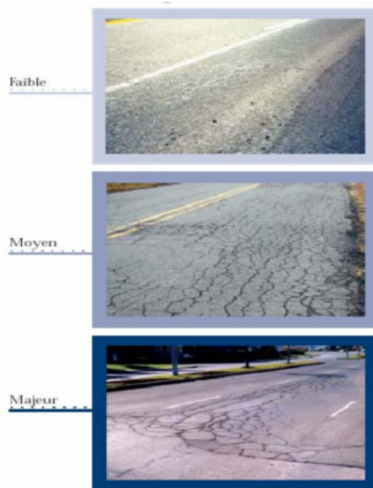
Figure I-17 : Fissures en carrelage
